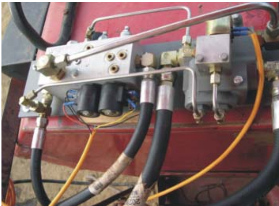
Figure 20. Hydraulic control system
